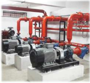
Fire Fighting Pumps
