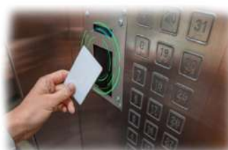
Elevator Access Control
