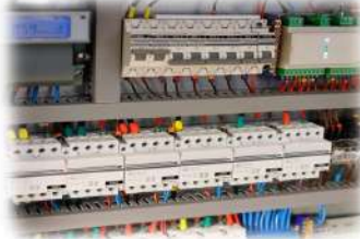
IOT / BMS Control Panel
