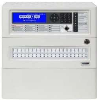
Conventional Control Zone Panel
